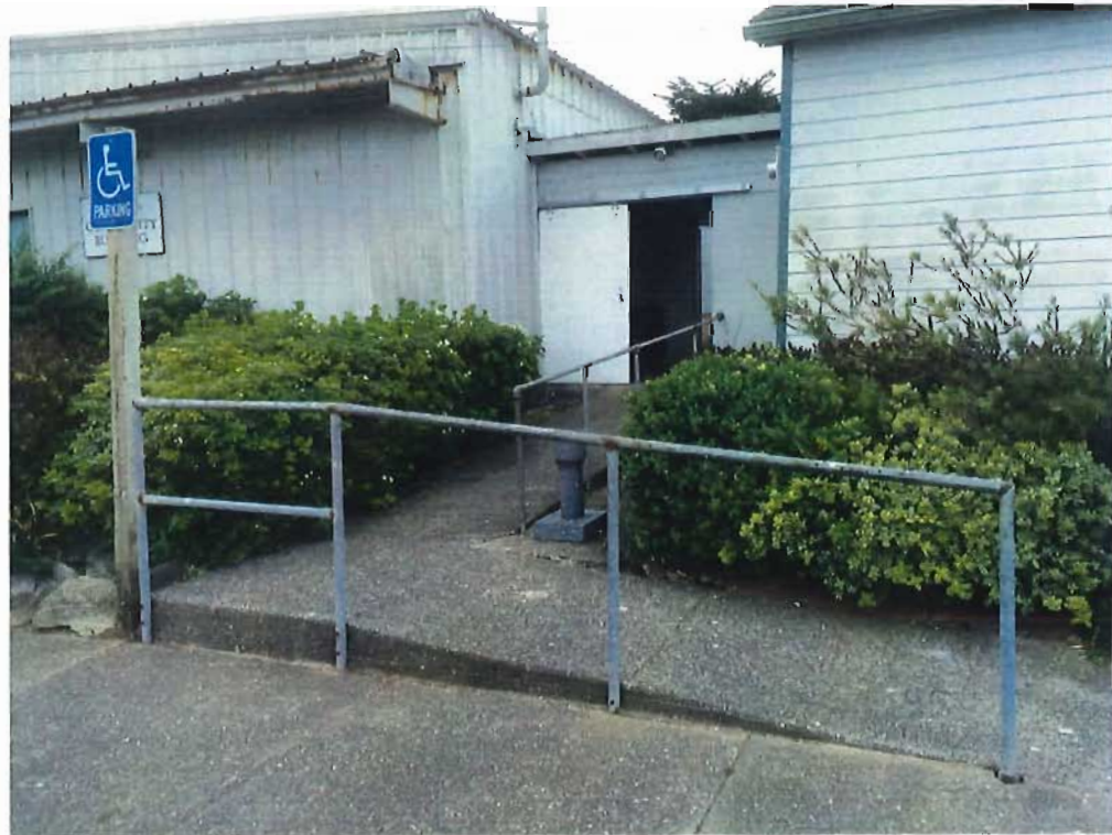
NON-COMPLIANT ADA RAMP
