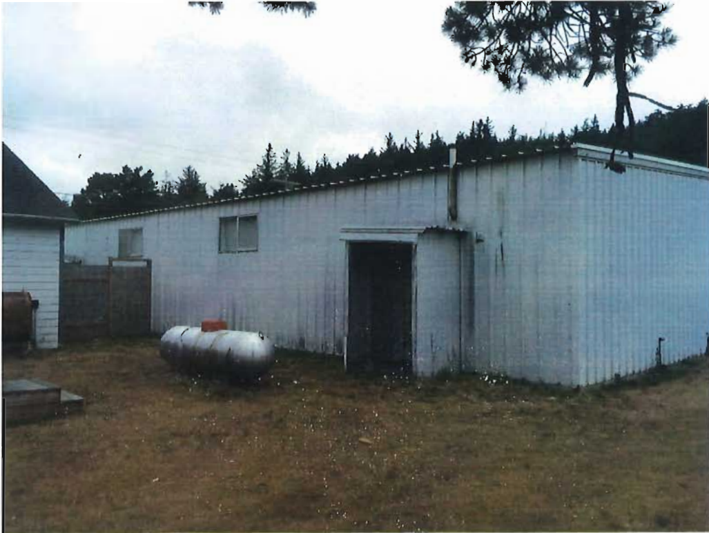
BUILDING NEEDS GUTTERS
