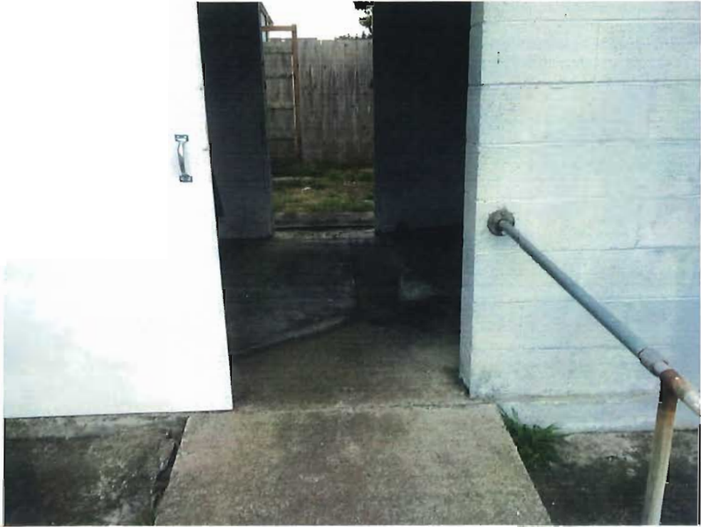
SUBSTANDARD SERVICE ENTRY
