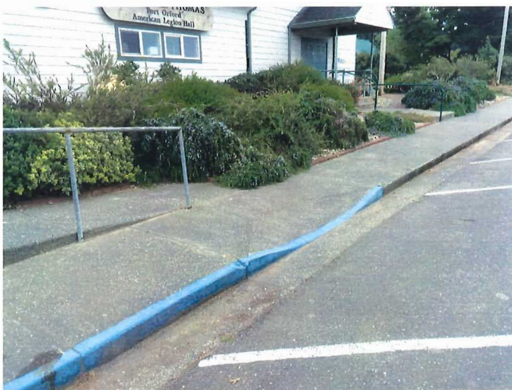
ADA ACCESS – NON-COMPLIANT
