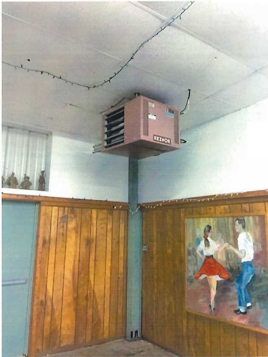
NOISY UNIT HEATERS
