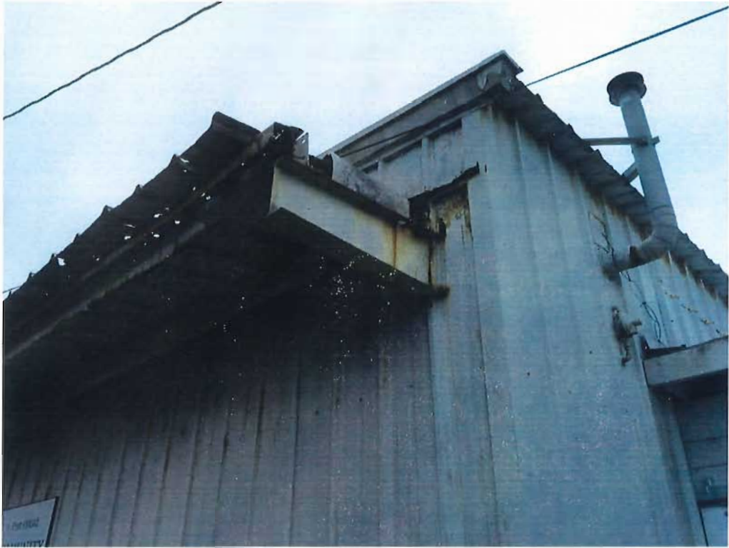
ROTTED ENTRY CANOPY
